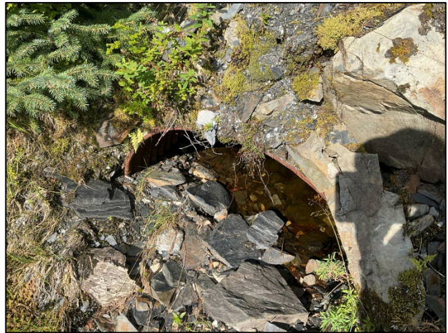
Figure 3.—Riprap at outlet of culvert causing backwatering at waypoint 972.
